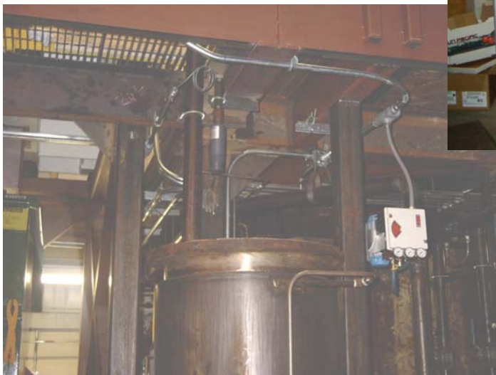
Holding Tank Ultrasonics
